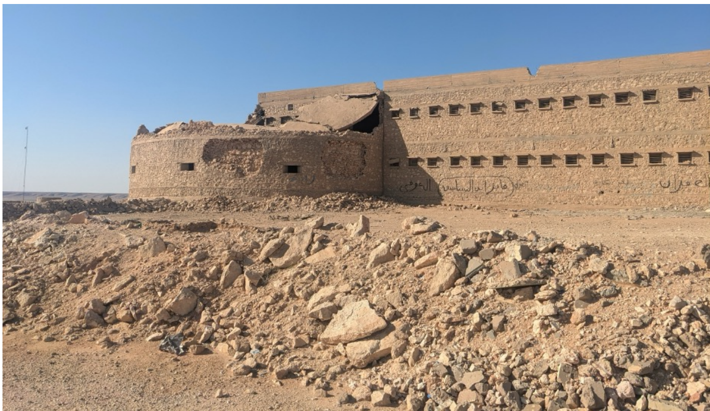
Figure 3. The caved-in roof of one of the towers of Saddam's prison at Salman in southern Iraq, viewed from the outside. Photographed January 2026 by the author.
